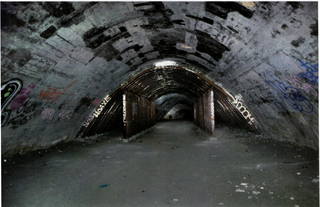
Reinforced section of Ouseburn culvert in Newcastle upon Tyne. The culvert was used as a public air-raid shelter during WWII. Photo Chris Rayner
